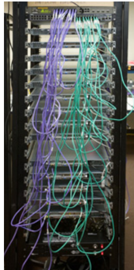
Testbed from the back. Lavender wires (left) are to the Gigabit data network; turquoise wires (right) are to the IPMI network. Power lines run inside a channel built in to the right edge of the rack.
